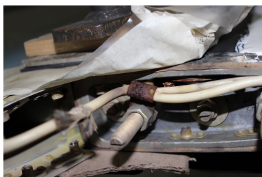
图4 旋翼内部导线包铁锈蚀 Fig. 4 Rotor internal wire wrapped iron corrosion
